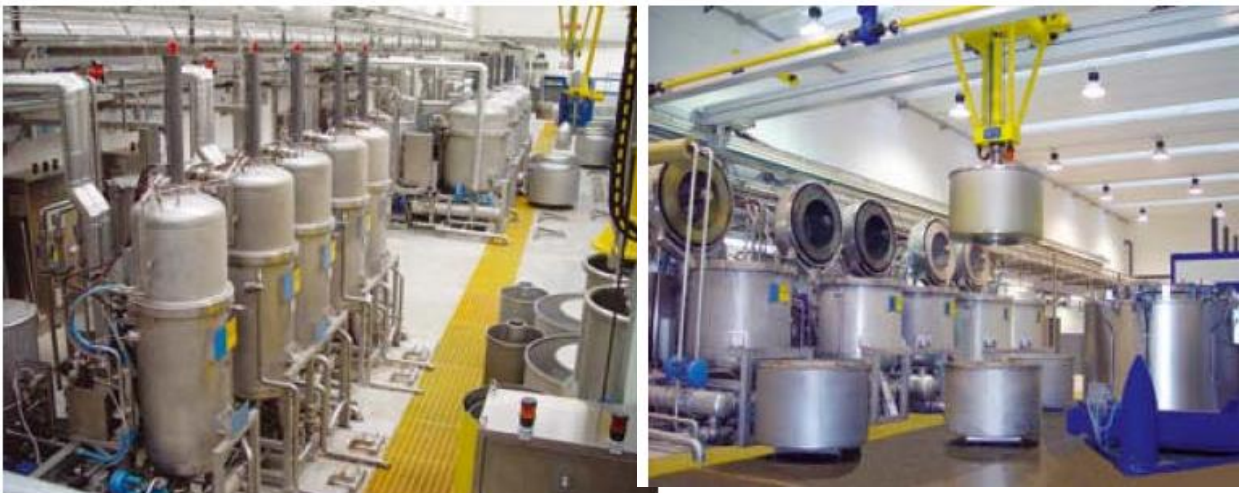
Photo: OBEM automated loose stock and top dyeing
